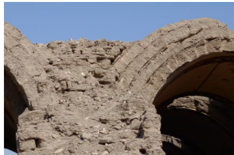
Figure 3. The adobe vault of the storeroom of the Ramesseum temple composed by four courses, the filling between the adjacent vaults can also be noticed.
