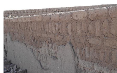
Figure 15. Many symptoms of damage in the storerooms of Sety I and the Ramesseum temples (a) cracking, (b) partial collapses, (c) holes widening, (d) erosion, (e) plaster detachment and (f) restoration using incompatible materials.
