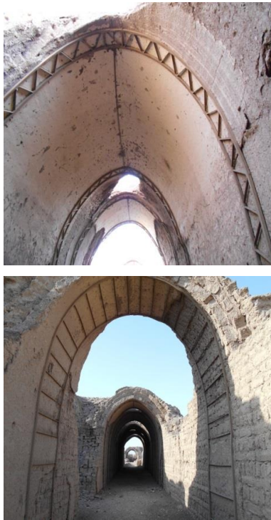
Figure 29. Two forms of the steel supporting structures used as strengthening interventions in the Ramessesum storerooms.
