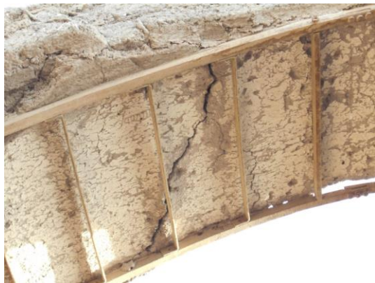
Figure 30. Large cracks at places of strengthening intervention.
