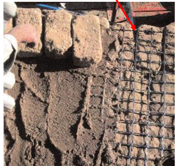
Figure 32. The application of polymer grids between adobe wall courses in Shunt el-Zebib in Abydos.
