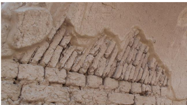
Figure 2. Mud-bricks laid tilted in an ancient Egyptian barrel vault (in the storerooms of the Ramesseum temple).
